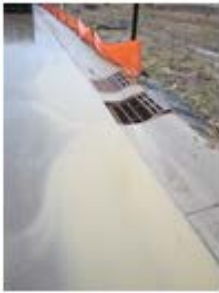
Sediment from construction site
