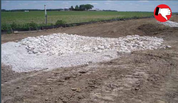
Check dam is much bigger than necessary. Wasted material, wasted money, can cause flooding, and will be much more difficult to remove.
