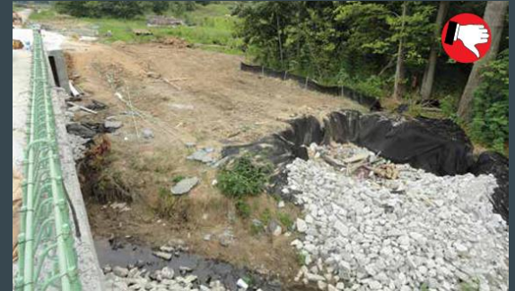
Keep construction debris contained in designated areas, away from hot spots and BMPs.
