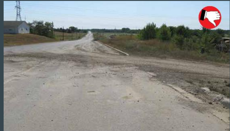
Insufficient #2 stone on construction entrance. Tracking onto public roadway. Mud tracked onto paved roads becomes a safety issue.
