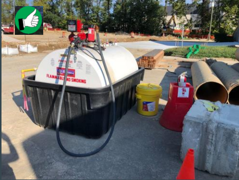
Fueling operations are located in a secondary containment to contain any spills or leaks.
