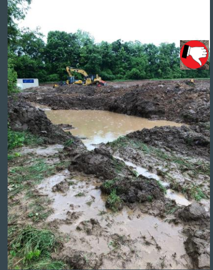
A poorly constructed sediment basin
