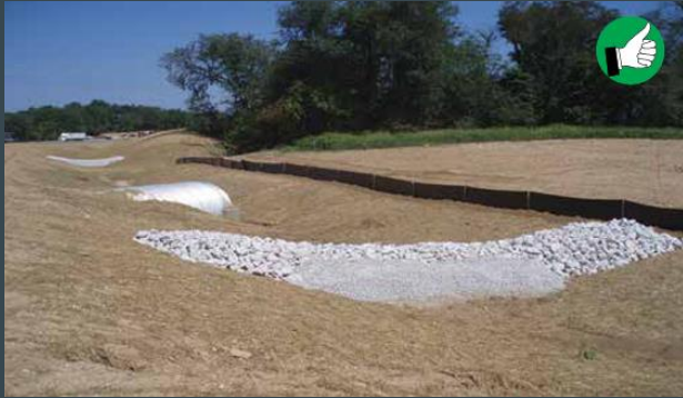
Check dam shaped correctly with low weir in the middle and tied into the slopes.
