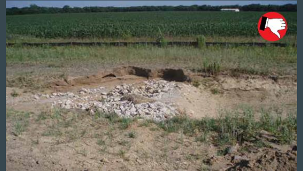
Check dam not shaped correctly causing water to bypass dam and erode slopes.
