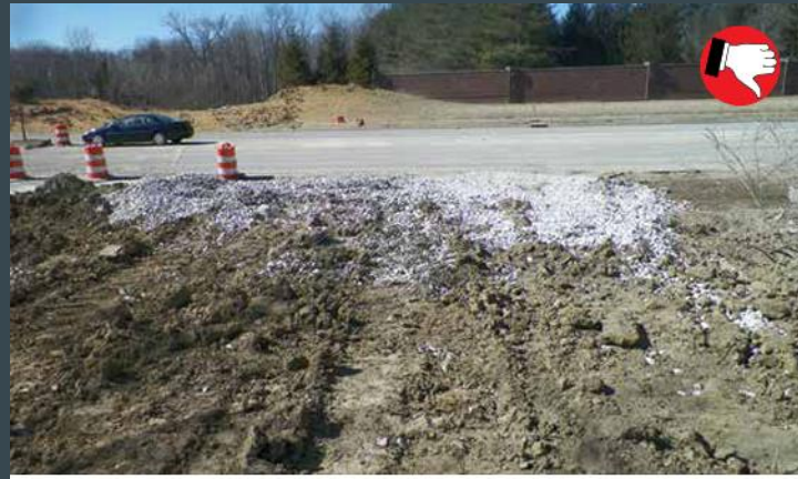
Construction entrance not the minimum 50' long. Tracking onto the roadway will become a safety hazard.
