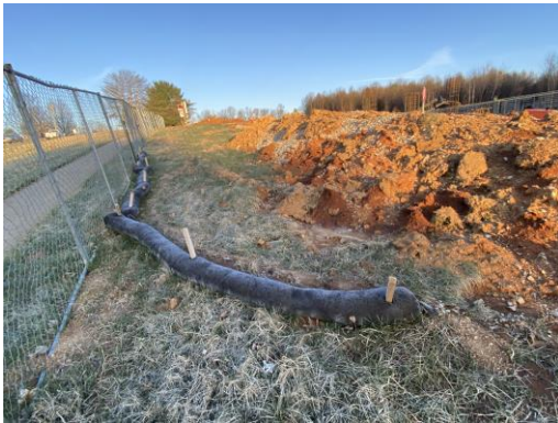
On slight slopes, straw wattles or coir logs with J-hooks can prevent sediment from leaving the site. They must be trenched in properly!
