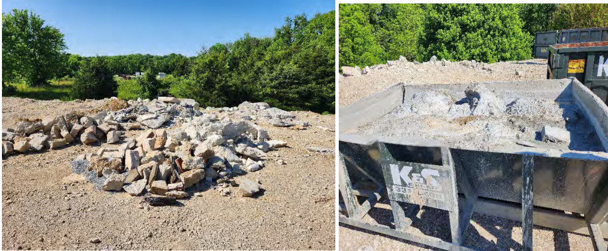
Photo 6. Concrete washout debris used to fill Sinkhole 'B'
