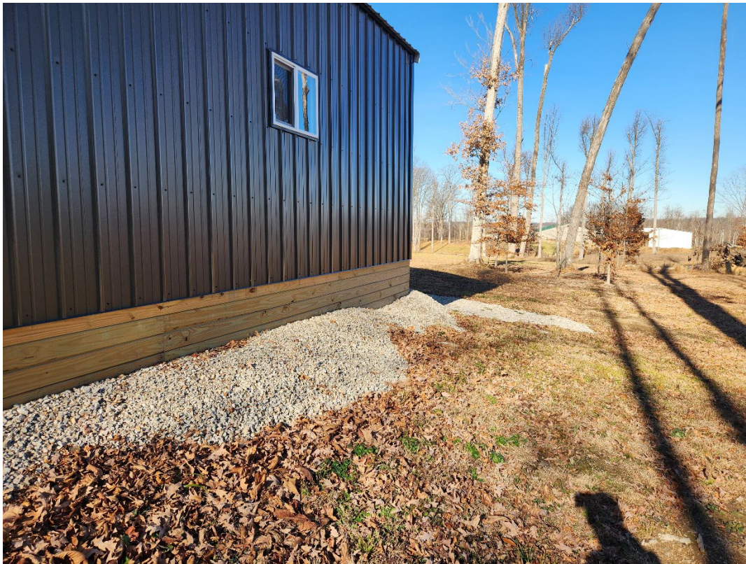
Photo 4 – Facing North (northeast side of building that encroaches rear setback)
