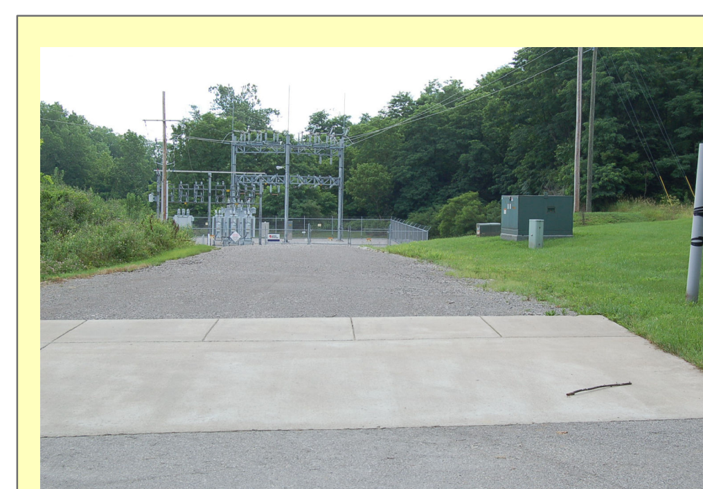
Small electric substation just north of the property.
