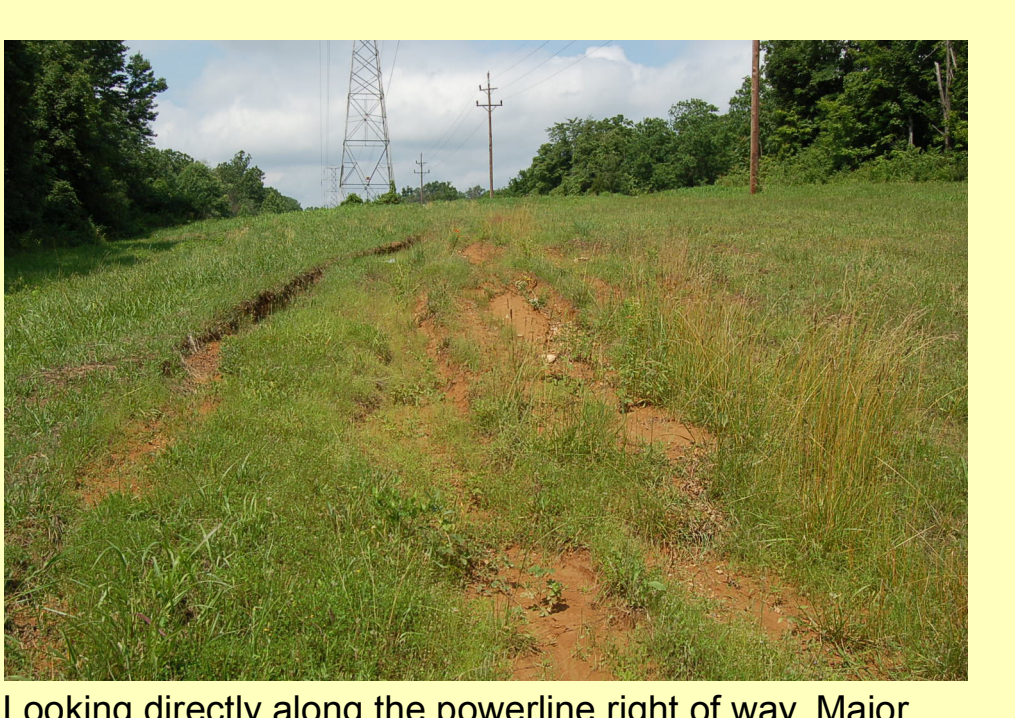
Looking directly along the powerline right of way. Major erosion on this slope, some ruts are a couple feet deep and wide.
