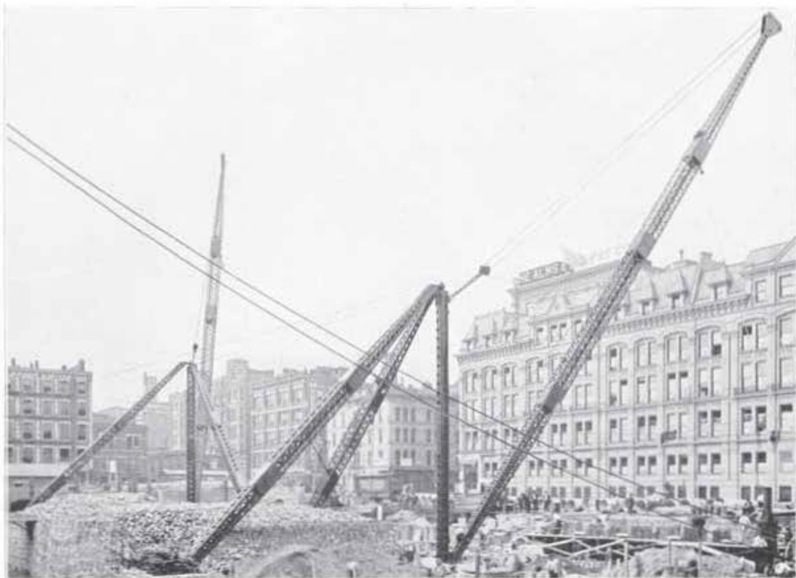
View of two Bedford Stiff-Leg Steel Derricks on construction work. These derricks are of 20-ton capacity, having 40-foot masts and 100-foot booms
