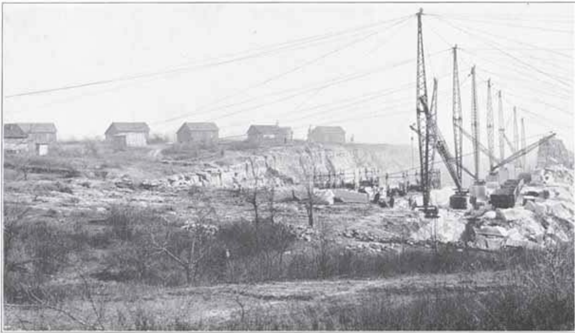
Seven 30-ton Steel Derricks, Dark Hollow Quarry, Consolidated Stone Co., Bedford, Indiana
