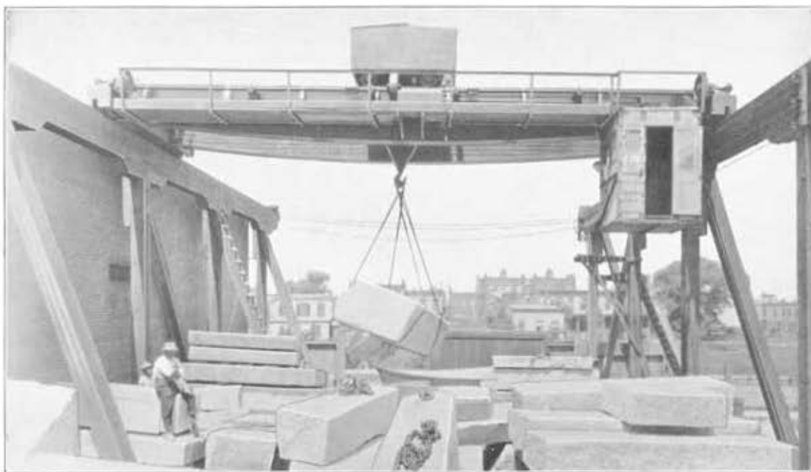
Tedeschi & Tedeschi, Long Island City, New York. 20-ton 39' span three-motor Electric Crane
