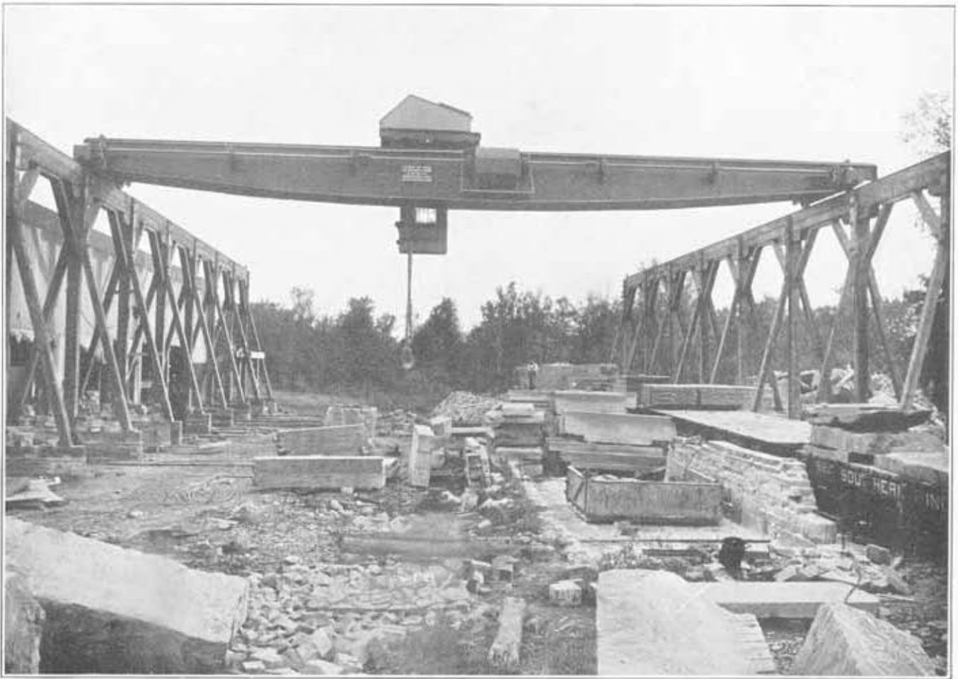
Shea & Donnelly Company, Bedford, Indiana, using a thirty-ton two-motor 70' 0" Span Bedford Electric Traveling Crane
